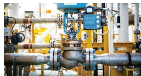
Emergency Shutdown Valve
